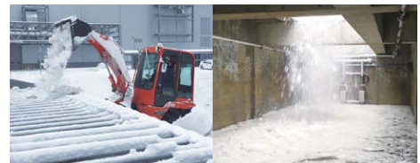
Snow use pit (left: Input port; right: pit interior)
