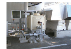
Heat pump type electric heating equipment installed at the factory
