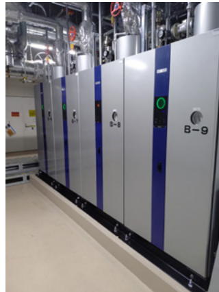
Used to preheat steam boiler feedwater
