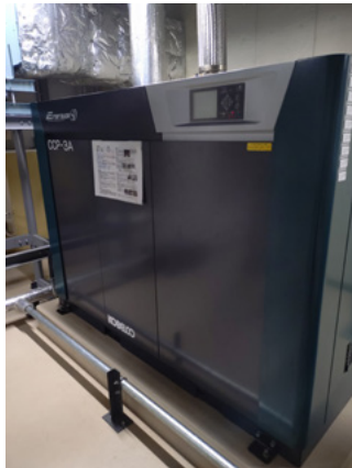
Steam-driven air compressor
