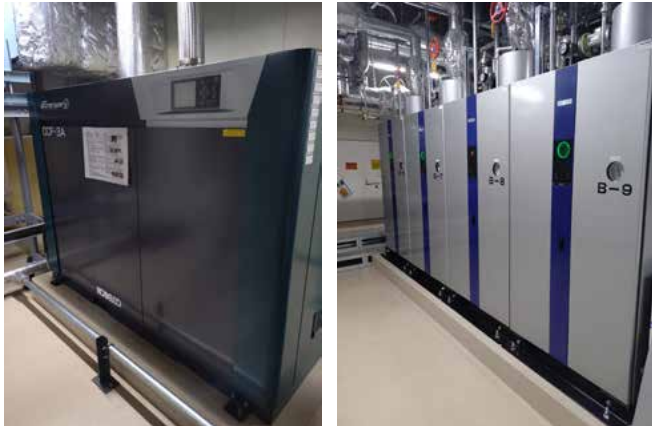
Steam-driven air compressor
